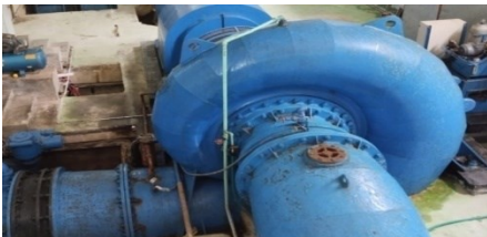
Gambar 1. Turbin francis PLTM Taluda'a
